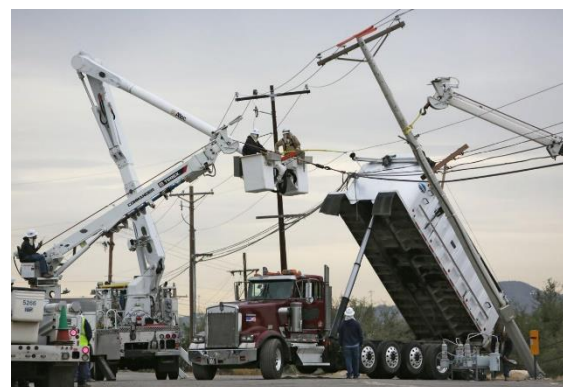
Survey work areas for overhead power lines before lifting any dump bed.
